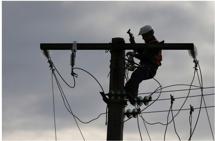
A technician works on an electrical power pylon during the maintenance of high-tension electricity power lines in Epinoy, near Cambrai, France, October 27, 2015. Rossignol/Reuters
