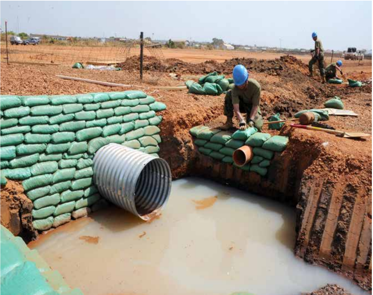
A team of engineers with the United Nations peacekeeping mission assists the government of South Sudan with road construction activities (February 2012).
